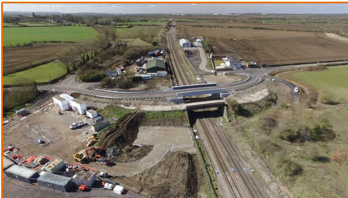
Aerial photo showing the location of the former Shrivenham Station, the Victoria Tavern on the far right, the new Railway Bridge being installed in 2016. Photo by Neil B. Maw
